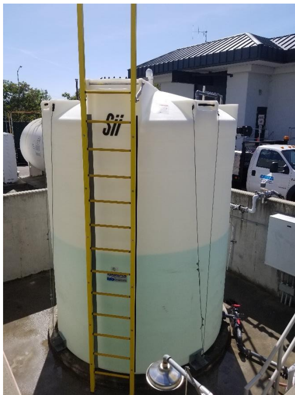
Recently Installed Nitrate Solution Bulk Chemical Storage Tank
