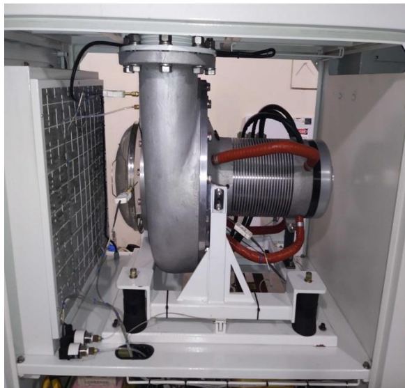
Blower Core Prior to Removal for Factory Maintenance
