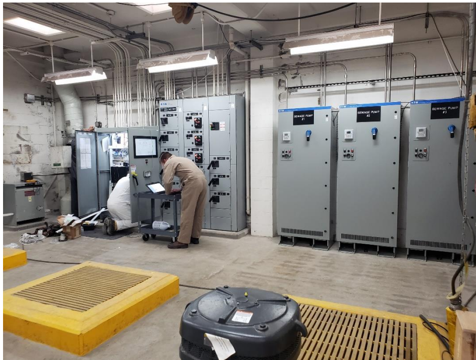
Newly Installed Motor Control Center, Control Panel, and Variable Frequency Drives at the SQPS
