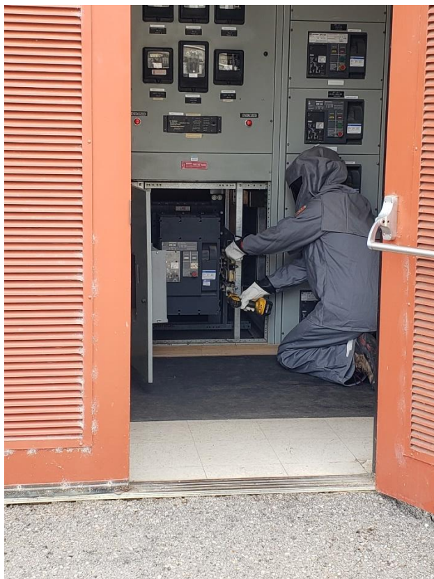
Switchgear inspection being performed
