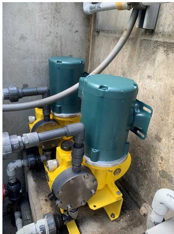
Refurbished Nitrate Solution Injection Pumps
