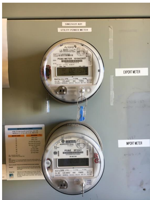
Power export meter to track the energy being sold to MCE
