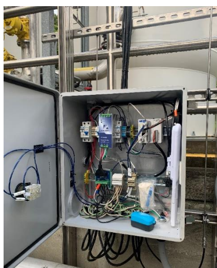
H2S Sampler Control Panel
